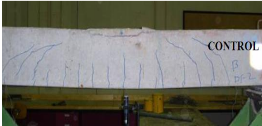
Figure 16: Crack pattern for control beam, group-1_ (Nadeem A.S 2009) (Experiments)
