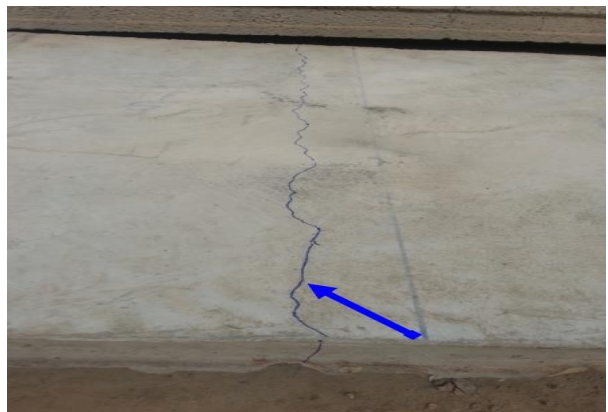
Figure 12: Panel 1 Cracks Pattern
