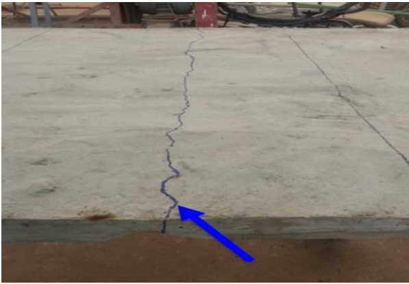
Figure 13: Panel 2 Cracks Pattern
