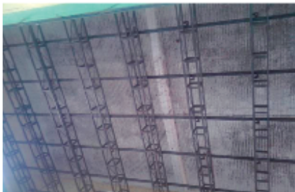
Plate (3): Lattice Box Girders lift to position, with purlins fixed on it just below the defected concrete roof.
