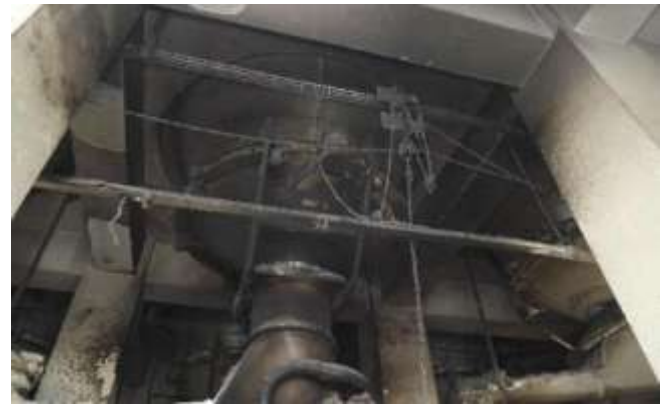
Figure 5 Wheat flour bins at section B (Explosion Zone)
