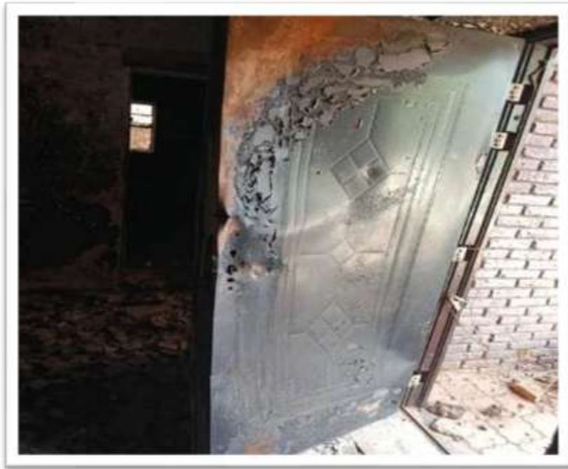
Figure A .11: Metal door with maintained overall integrity and coating deterioration
