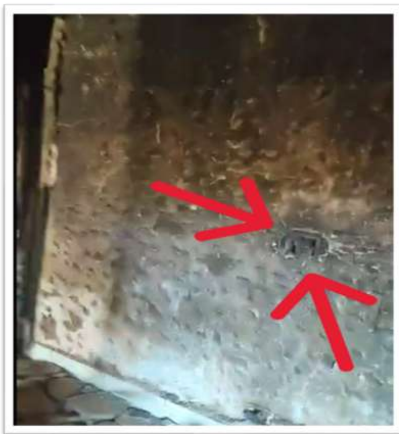
Figure A .14: Melted electrical switch cover in kitchen area
