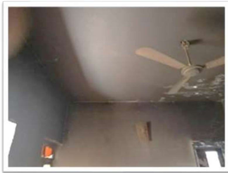
Figure A .13: Ceiling fan mounted at the centre of the room 1 with visible soot but no apparent distortion
