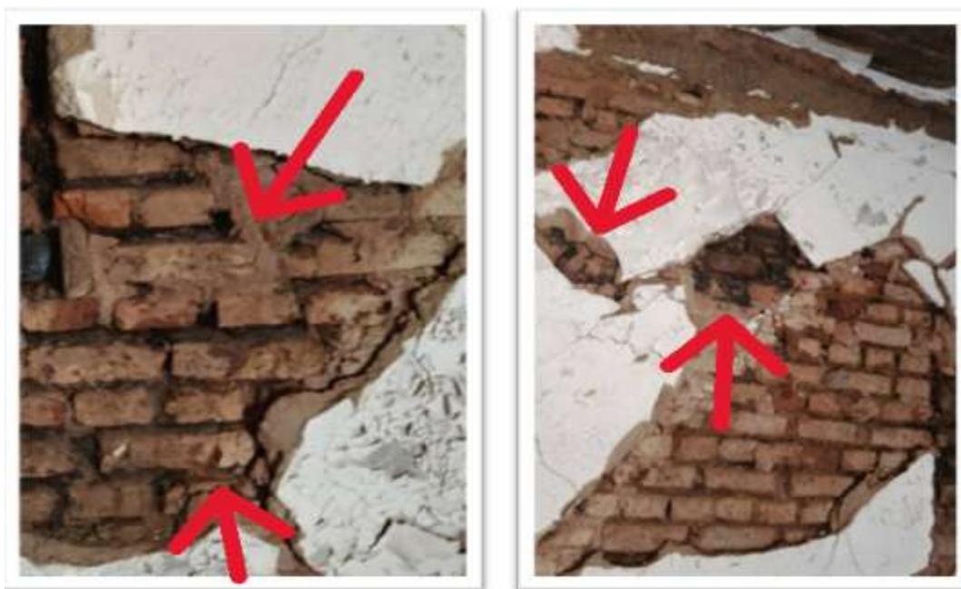
Figure A .8: Discoloured mortar joints in brick walls of room 3
