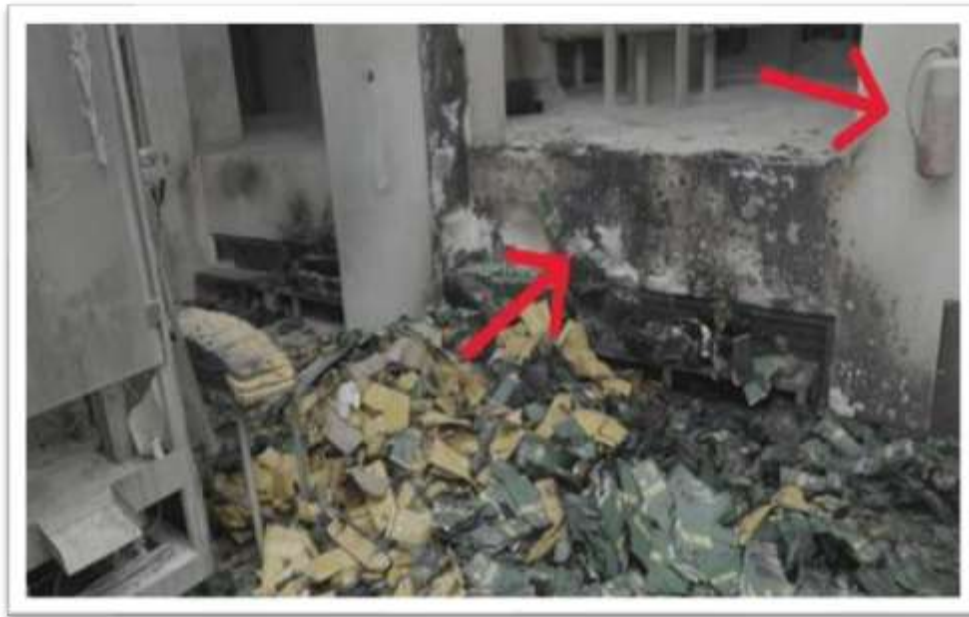
Figure A .4: Destroyed paint of concrete members adjacent to flour bins [24]
