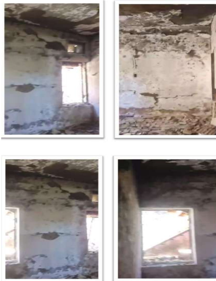
Figure A .16: Photos captured from video of room 2 showing plaster and paint damage with further assessment needed
