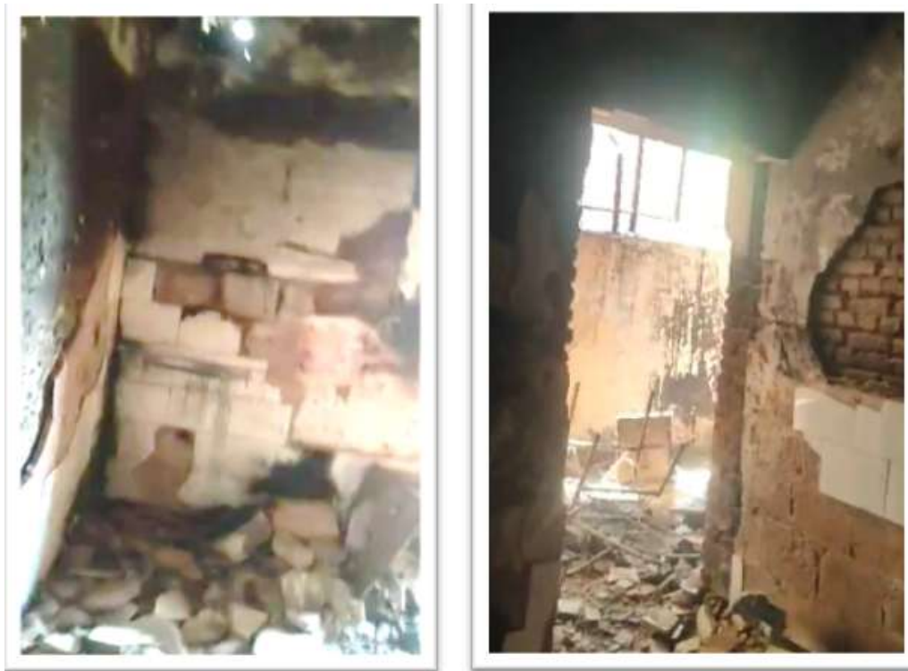
Figure A .15: Kitchen area showing significant structural damage with characteristics most likely consistent with explosion and fire effects
