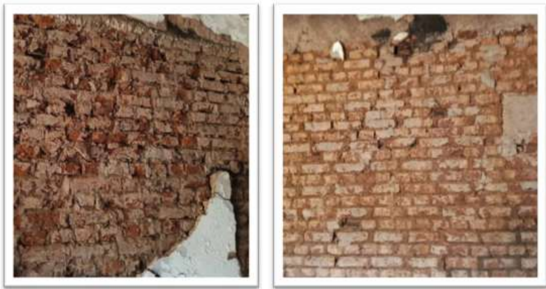
Figure A .7: Exposed brick masonry with relatively intact structure and plaster spalling at different parts inside room 3
