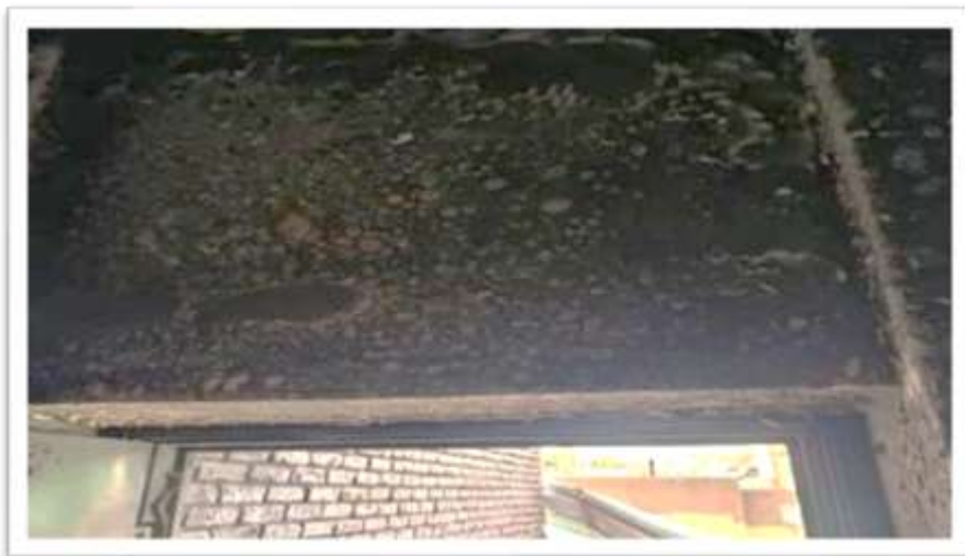
Figure A .6: Bubbled paint with soot above the steel door
